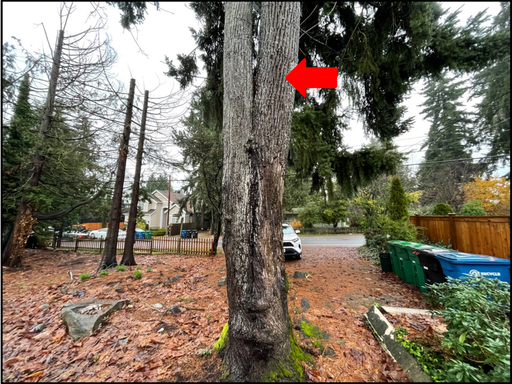
Photograph 4. The base of tree 101 with a poor union. The southern stem (red arrow) should be reduced to mitigate the hazard posed by this tree to the adjacent house.
